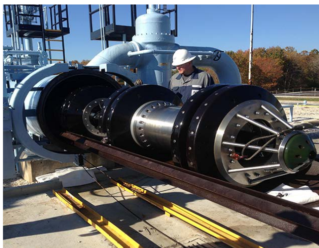
A smart pig is pulled from a receiving trap to complete an inline inspection.
